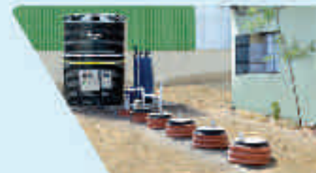
STP's Sewage Treatment Plant
